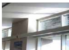
Daylight Redirecting Blinds (Daylighting Zone)
